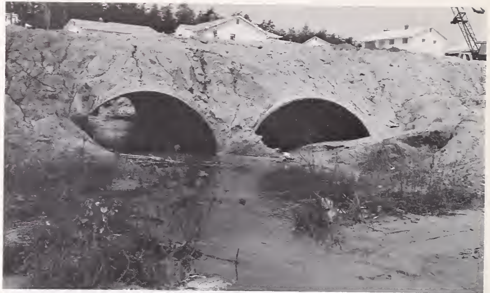
The runoff from this housing development pollutes the nearby stream.
